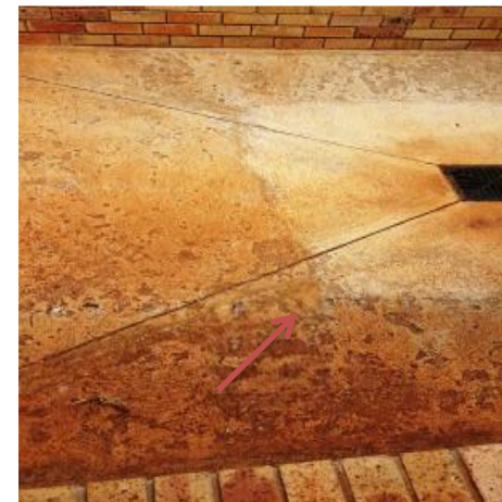
Picture 2: Honeycombing of concrete surface due to inferior concrete mix, at Midoroni Clinic (Limpopo)
