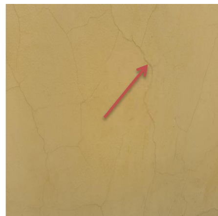
Picture 3: Hairline crack around entire external wall, due to inferior plaster mix, at Thembisa Hospital (Gauteng)
