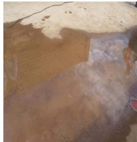
Picture 1: Ponding at surface bed due to poor sloping of surface at Vaal Bank Clinic (Eastern Cape)
