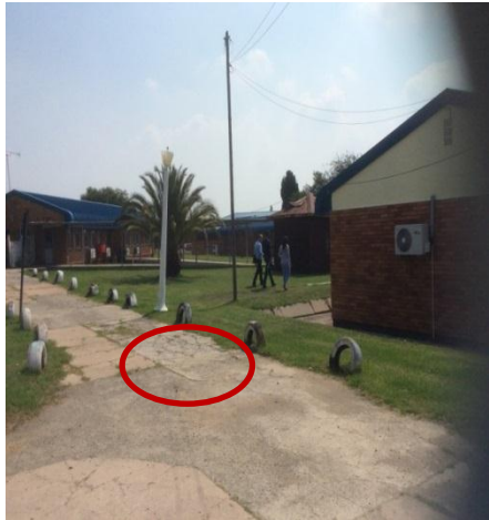
Picture 5: Crack on the pavement, due to inferior concrete mix, at Evander Hospital (Mpumalanga)
