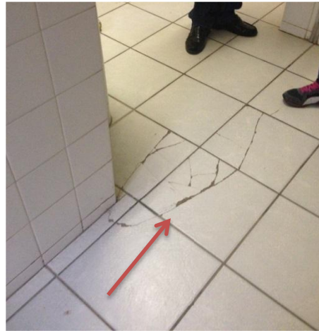
Picture 6: Newly installed tiles already cracked at Excelsius Nursing College (North West)
