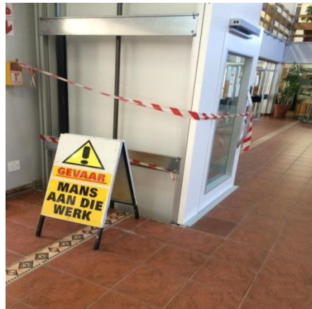
Picture 8: Elevator not complete due to poor quality work done, at CH Baragwanath Hospital (national facility)
