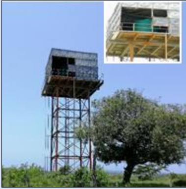
Manzengwenya KwaSonto project: 5kl tanks were placed in existing structure and 30kl tank was not in place.
