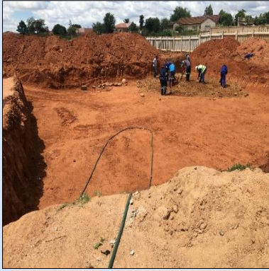
Moshate project: Project was incomplete on 10 December 2020, with contractor still on earthworks in preparation for the foundation for steel tank base
